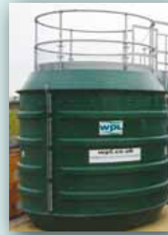
HiPAF Compact installed above ground (left)
