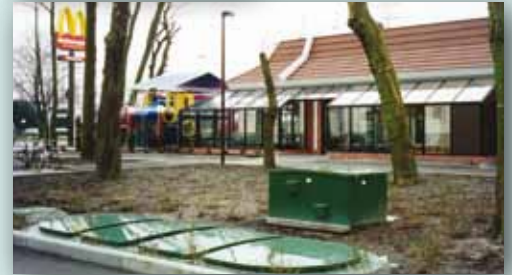
HiPAF Midi installed at an out of town fast food restaurant (below)
